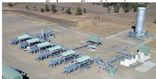
<New gas processing facility (Unit 3)>
